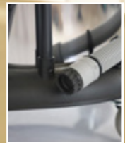
DRAINPIPE TO DISCHARGE COLLECTED WATER
