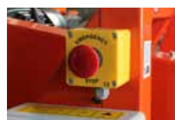
EMERGENCY PUSH BUTTON
