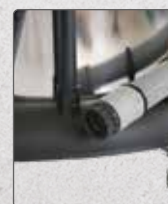
DRAINPIPE TO DISCHARGE COLLECTED WATER
