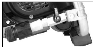
water supply closed (valve lever across)
